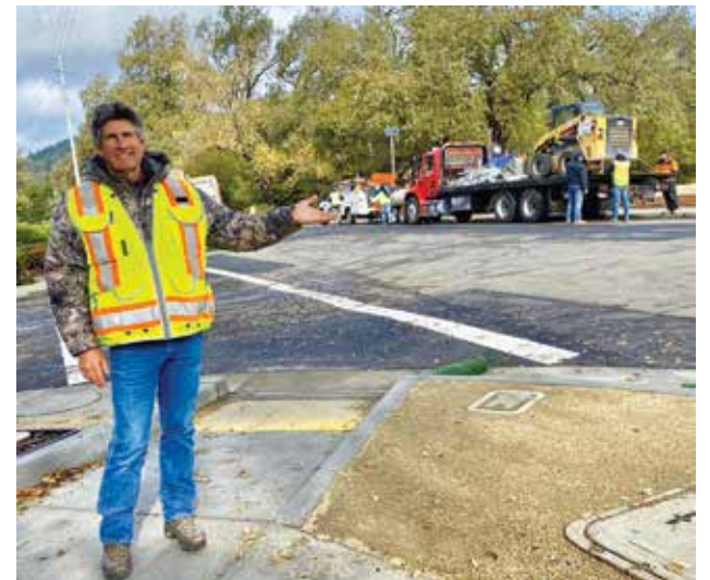
Charlie Young, project manager, supervised as the last equipment was loaded to be hauled away. (Photo by Julie Kiil)
