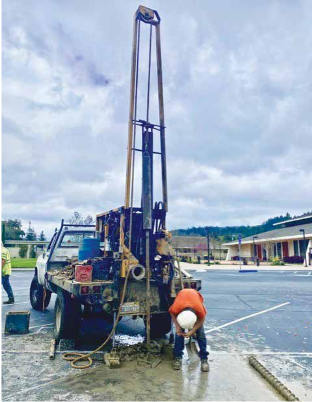
The solar panel project at Oakmont parking lots moved forward with a Terracon Consultants field geologist and California Geotech on location drilling to collect soil samples to help determine construction design at the three recreation centers' lots. The work did not collide with parking needs, as the recreation centers were closed. (Photo by Julie Kiil)
