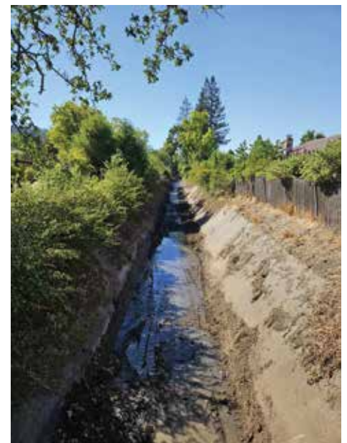
On Tuesday, Sept. 3, the Sonoma County Water Agency started dredging a section of Oakmont Creek that runs between Oakmont Drive and Wild Oak Drive, which should improve the flow once the rainy season begins again. These photos by resident Sherri Hoefling show what the creek looked like before and after dredging.
